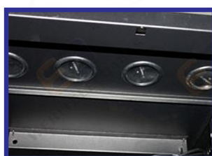
Wiring round holes
